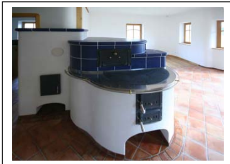
Pic 9 – Accumulator stove combined with kitchen stove situated in the centre of the house on the ground floor. It can be loaded with 10kg of wood and lasts heated for 24 hours - in this case the wall heating in the ground and first floor halls is switched off.
