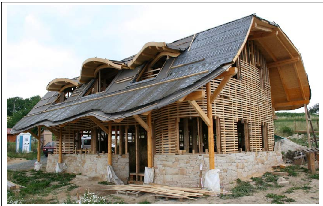
Pic 3 - Wooden construction of the family house made of natural building materials. This house will be insulated with 350mm (13.78 in) thick cereal straw bales pushed and pressed from inside into the wooden construction (for detailed wall construction please see picture 4). Roof of this house will consist of a shale roof part and an extensive green roof part at the top with lower slope. There will be an 80mm (3.15 in) air space under both roof covers.
