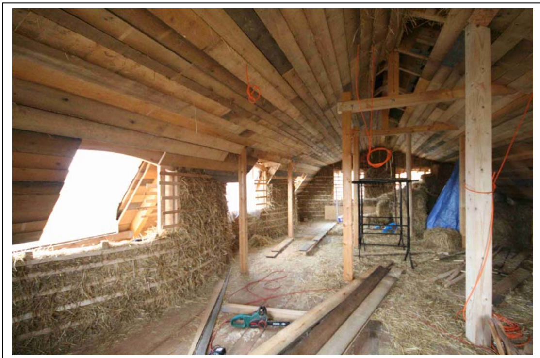
Pic 6 – The interior of the first floor with semi-finished walls and ceiling boards. On the left wall, vertical wood boards 24 mm (0.945 in) will be nailed to the horizontal wooden rods. On that will be placed a reed mat, low temperature wall heating and 20 - 30 mm (0,787 - 1,181 in) thick clay plaster made of clay from the building site.
