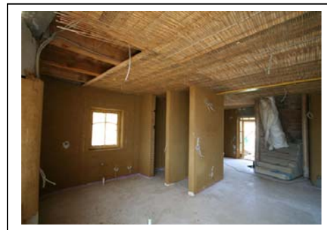
Pic 10 – Semi-finished ground floor. Enclosure walls are clay plastered with hot water heating inside. Ceiling is all-wood sheeted with ceiling boards, reed mat and clay plaster. Partition walls and sound insulation in the floor of the first floor are made of unfired bricks.
