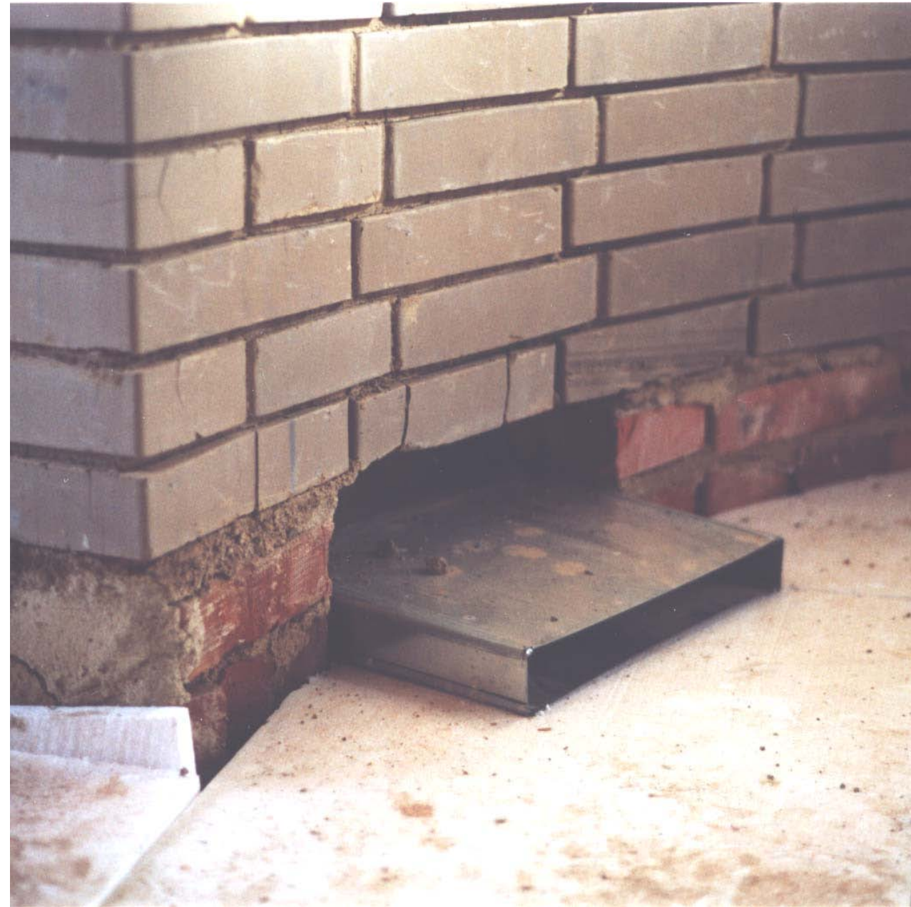
tube for warm or cold air joint into walls made from unburnt bricks
