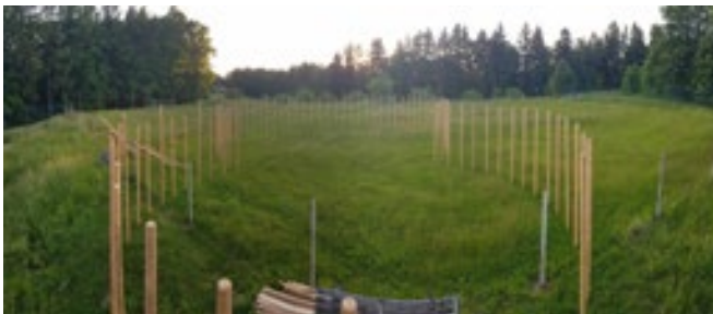
Place of construction and delineation of the building outline on the plot.
